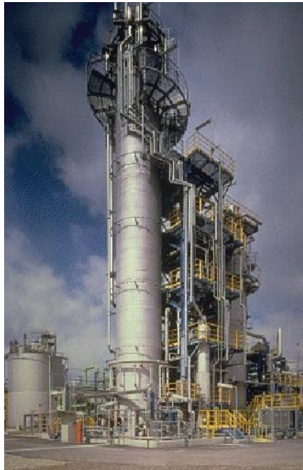
Figure 1.2 Hydrogen Peroxide Manufacturing Plant
