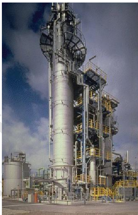
Figure 1.2 Hydrogen Peroxide Manufacturing Plant
